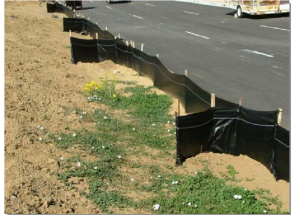
Photograph SF-2. When silt fence is not installed along the contour, a "J-hook" installation may be appropriate to ensure that the BMP does not create concentrated flow parallel to the silt fence. Photo courtesy of Tom Gore.
