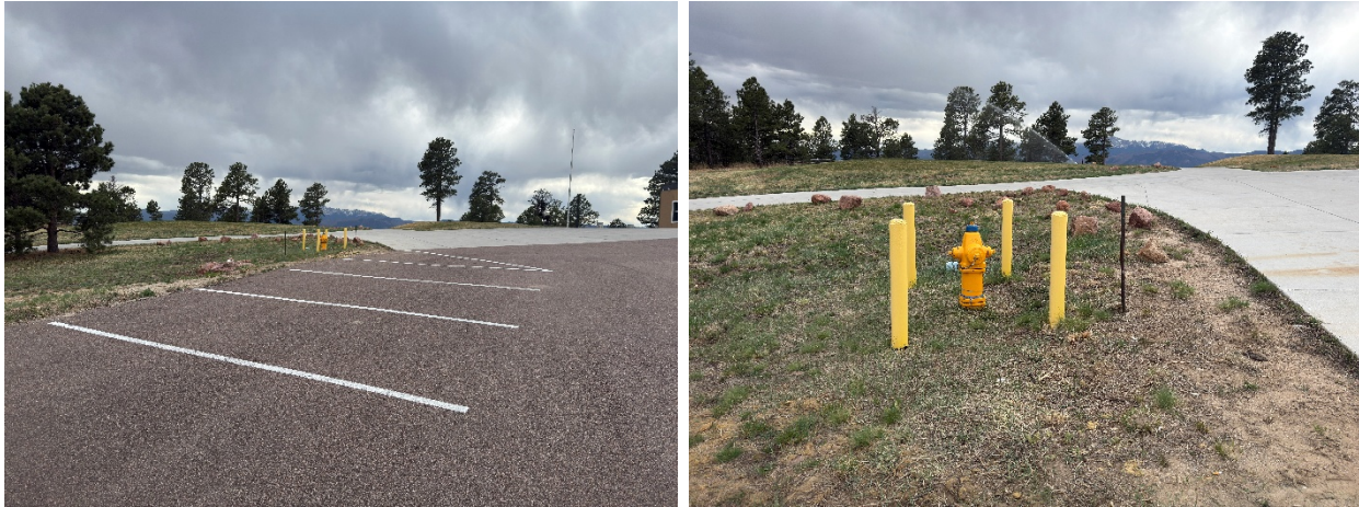
Figure 1: Existing Fire Hydrant at Clubhouse
