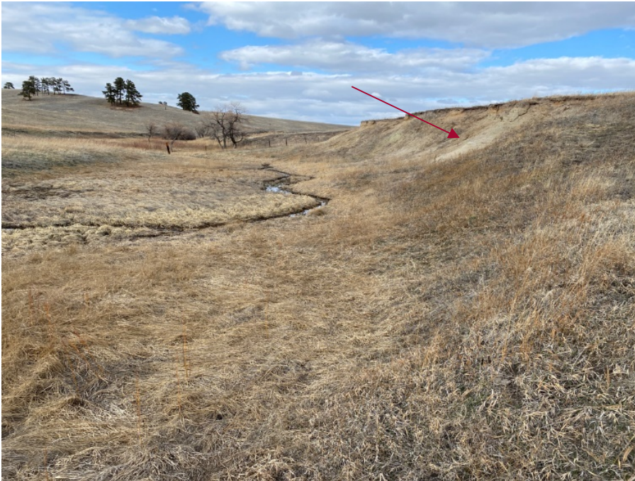
Photo 4 - Erosion on valley/terrace transition (slope on right). Note: Stable channel and floodplain
