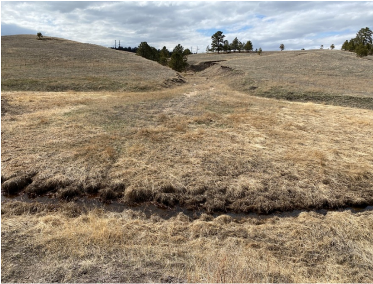
Photo 5 - Erosion at Cross-Section 4312 (slope on right).
