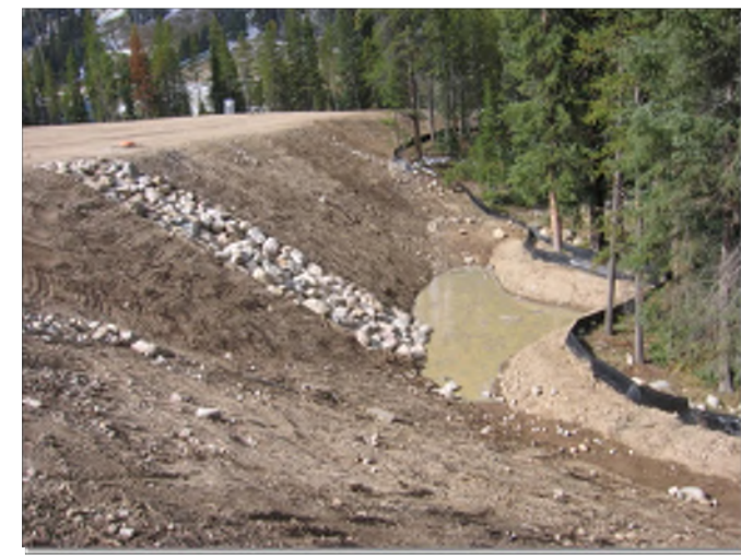
Photograph SB-1. Sediment basin at the toe of a slope. Photo courtesy of WVE.
