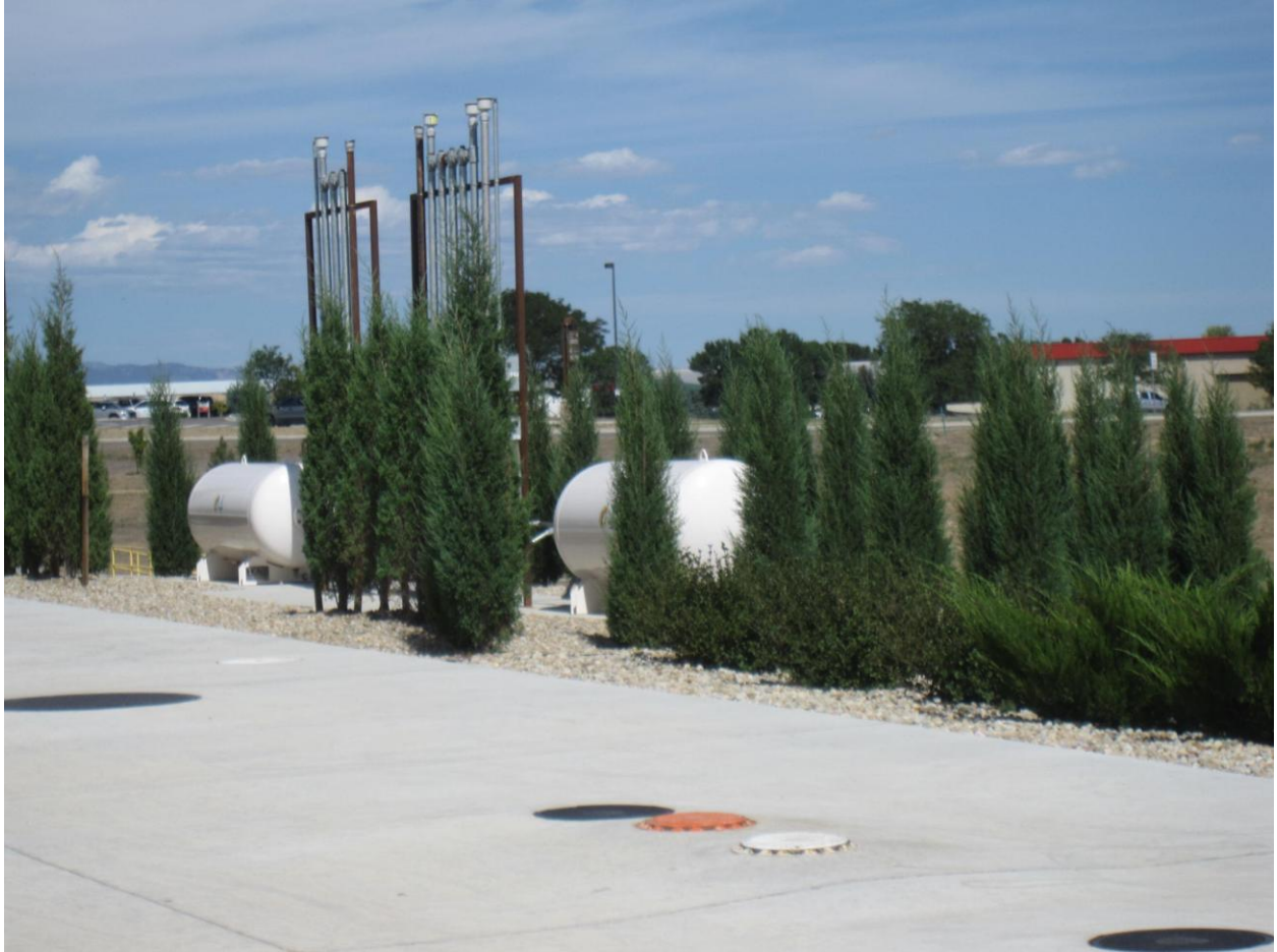
Photo 7. The proximity of upright and Pfitzner junipers pose a threat to the pressure tanks that serve the gas pumps. This is located at the Johnstown location.
