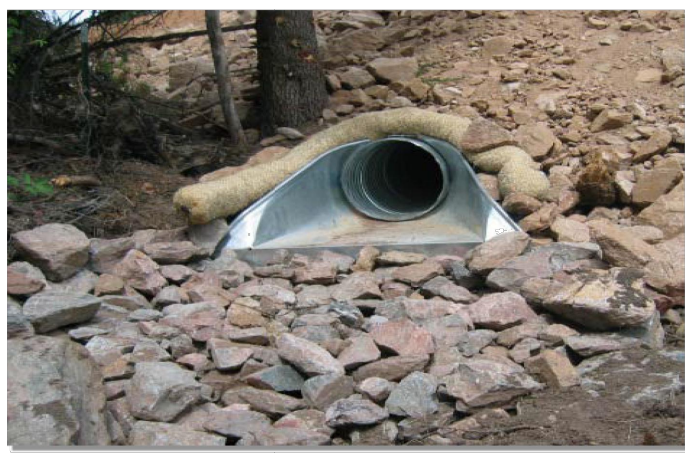
Photograph TOP-1. Riprap outlet protection.
