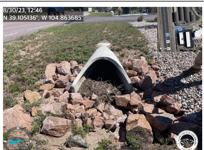
Photo 4: Clean out both flared end sections of culvert along Deer Creek Road.
