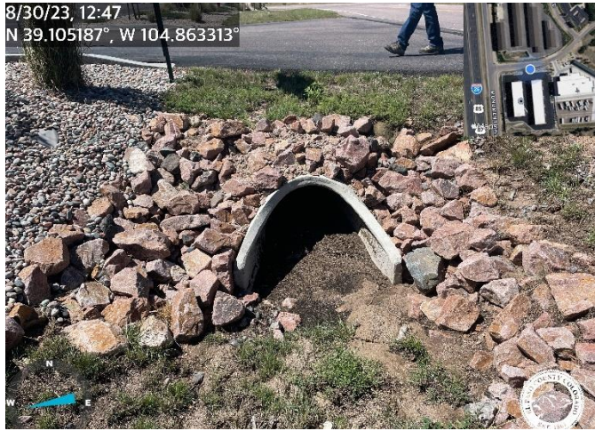
Photo 5: Clean out both flared end sections of culvert along Deer Creek Road.
