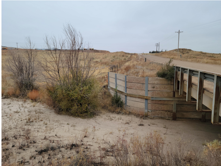
Figure 9: Creek Entrance under S. Franceville Coal Mine Rd, site shown in the distance to the South. Drainage path shown along roadside draining into the creek.
