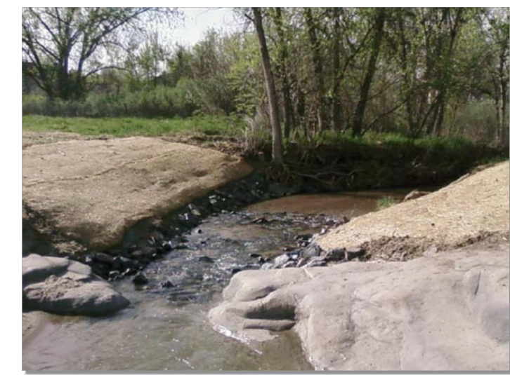
Photograph SS-1. Streambank stabilization using geotextiles following installation of a permanent in-stream grade control structure.
