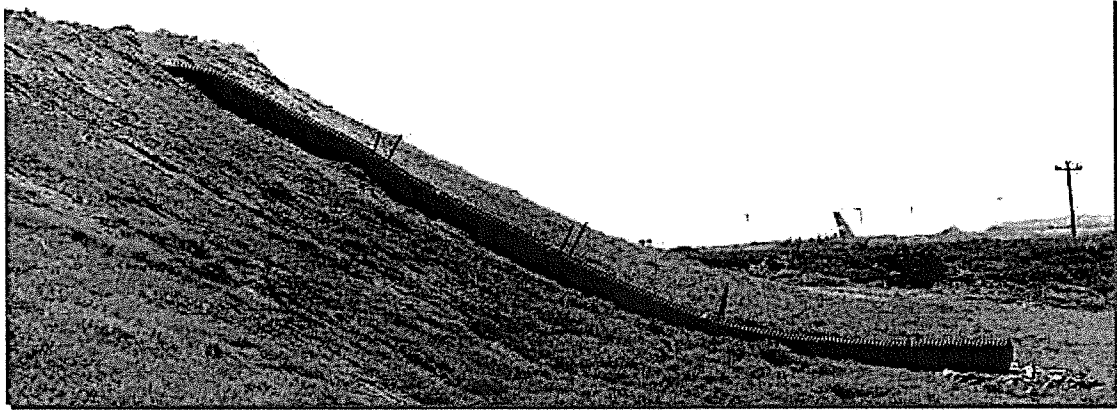
Photograph TSD-1. A temporary slope drain installed to convey runoff down a slope during construction. Photo courtesy of the City of Aurora.
