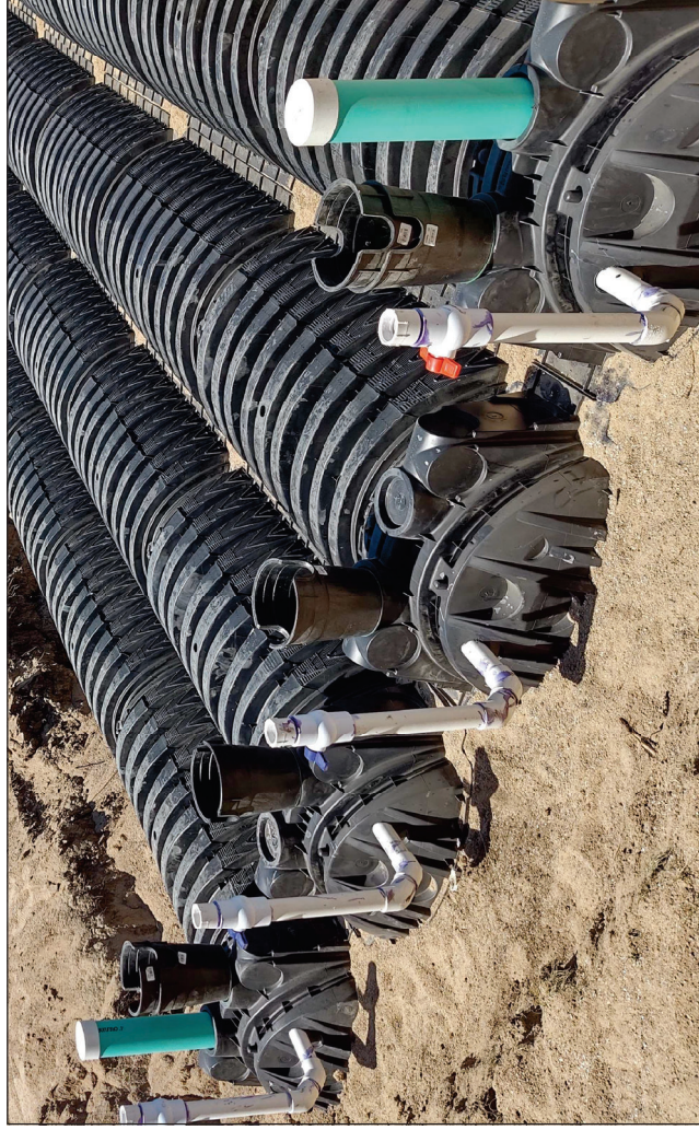
Typical Flush Port with Ball Valve (Ball Valve not Required in all Counties)
