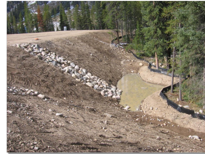
Photograph SB-1. Sediment basin at the toe of a slope. Photo courtesy of WVE.
