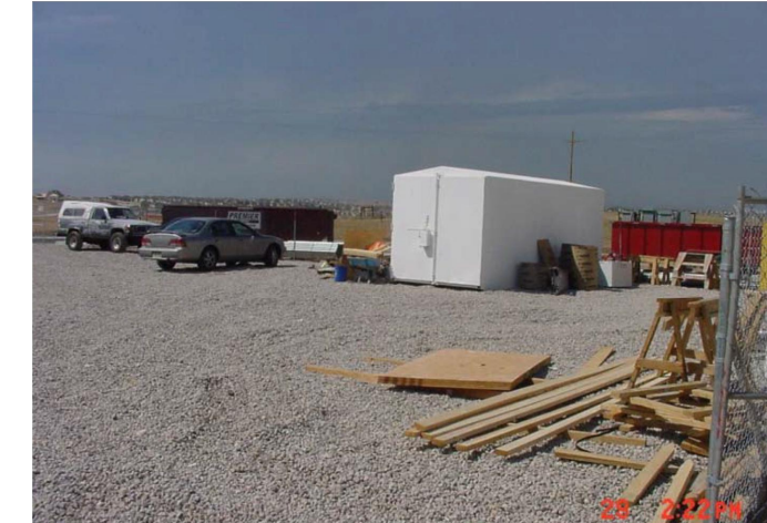
Photograph SSA-1. Example of a staging area with a gravel surface to prevent mud tracking and reduce runoff. Photo courtesy of Douglas County.
