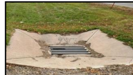
CDOT Type C Inlet in Depression
