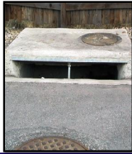
Denver No. 14 Curb Opening
