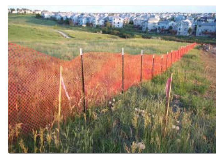
Photograph CF-1. A construction fence helps delineate areas where existing vegetation is being protected. Photo courtesy of Douglas County.
