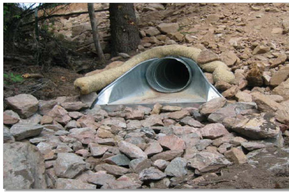
Photograph TOP-1. Riprap outlet protection.
