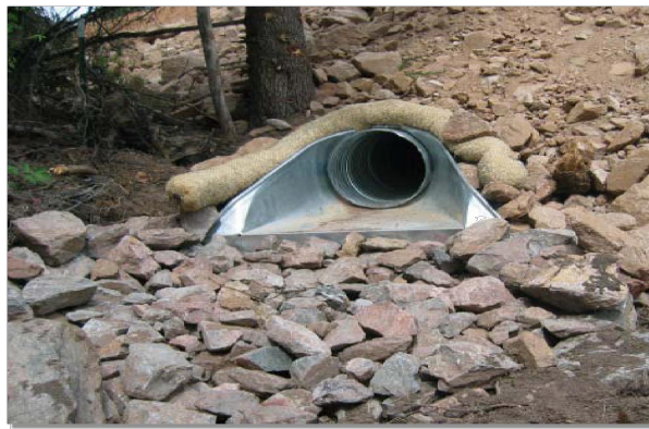
Photograph TOP-1. Riprap outlet protection.
