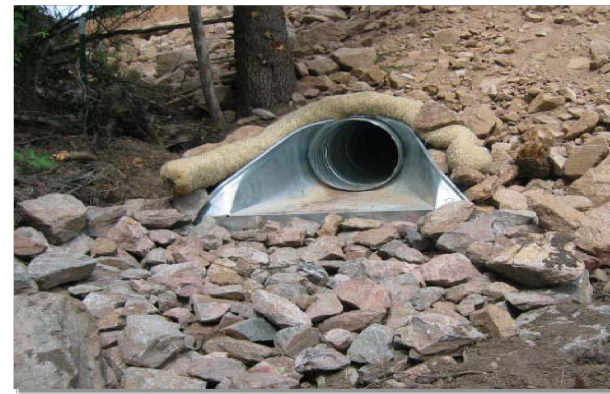
Photograph TOP-1. Riprap outlet protection.
