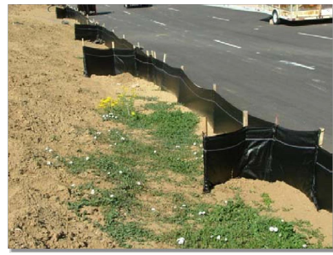
Photograph SF-2. When silt fence is not installed along the contour, a "J-hook" installation may be appropriate to ensure that the BMP does not create concentrated flow parallel to the silt fence. Photo courtesy of Tom Gane.
