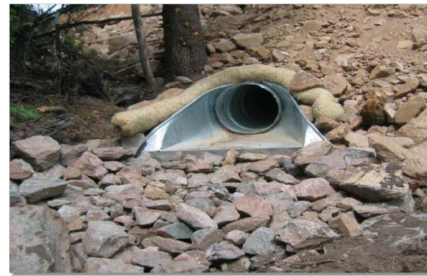
Photograph TOP-1. Riprap outlet protection.
