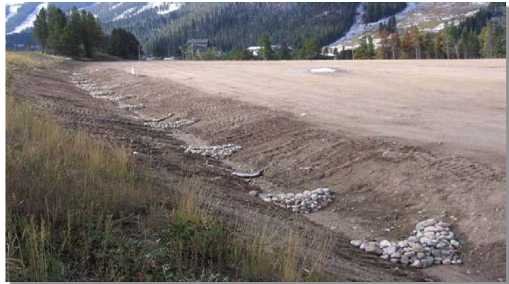
Photograph CD-1. Rock check dams in a roadside ditch. Photo courtesy of WWE.
