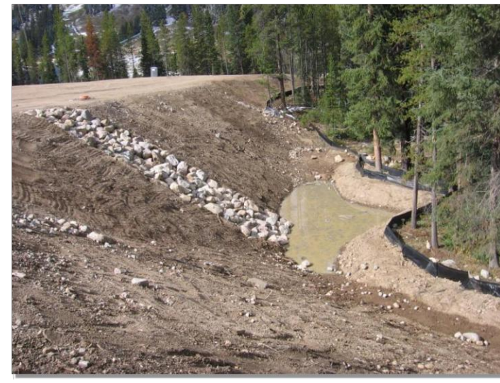
Photograph SB-1. Sediment basin at the toe of a slope. Photo courtesy of WVE.
