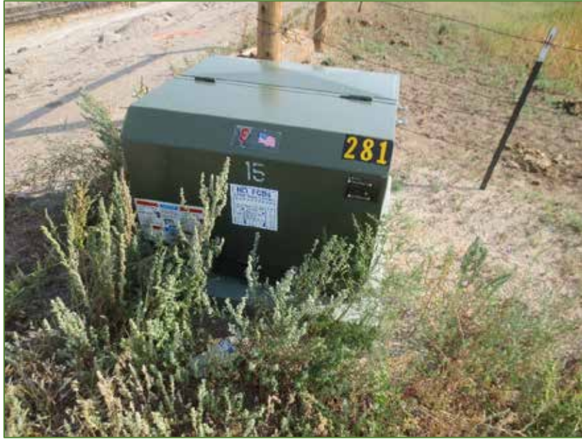
Pad-mounted electrical transformer.
