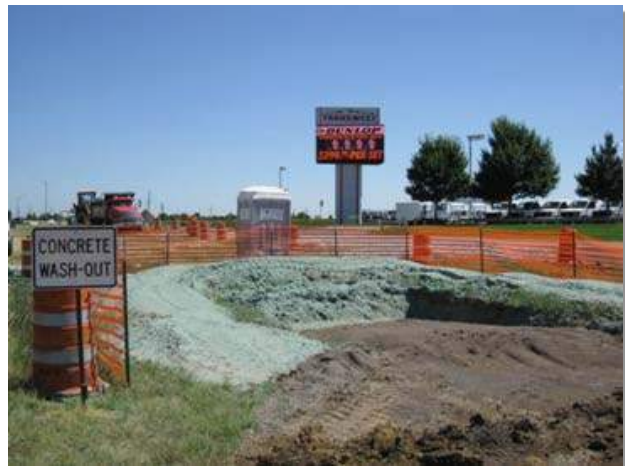
Photograph CWA-3. Earthen concrete washout. Photo courtesy of CDOT.
