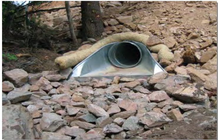
Photograph TOP-1. Riprap outlet protection.
