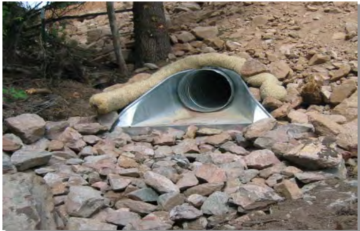
Photograph TOP-1. Riprap outlet protection.
