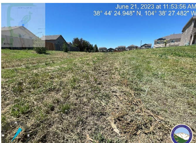
Photo 7: Clear and remove vegetative debris from swale upstream of pond.
