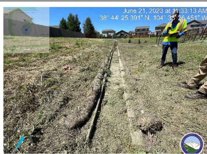
Photo 1: Low flow channel. Remove temporary control measures throughout and backfill to grade.
