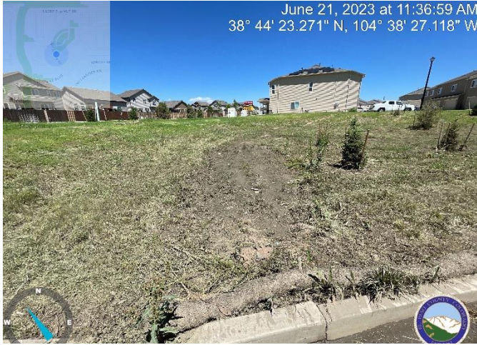
Photo 5: Reestablish maintenance access rd. and grade low spot for positive drainage. Remove trees from pond bottom.
