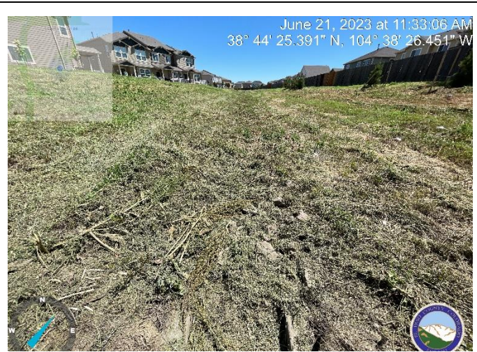
Photo 2: 9" D50 rip rap pad at north end of low flow channel needs to be cleaned and reestablished. Reference C4.6 of approved GEC
