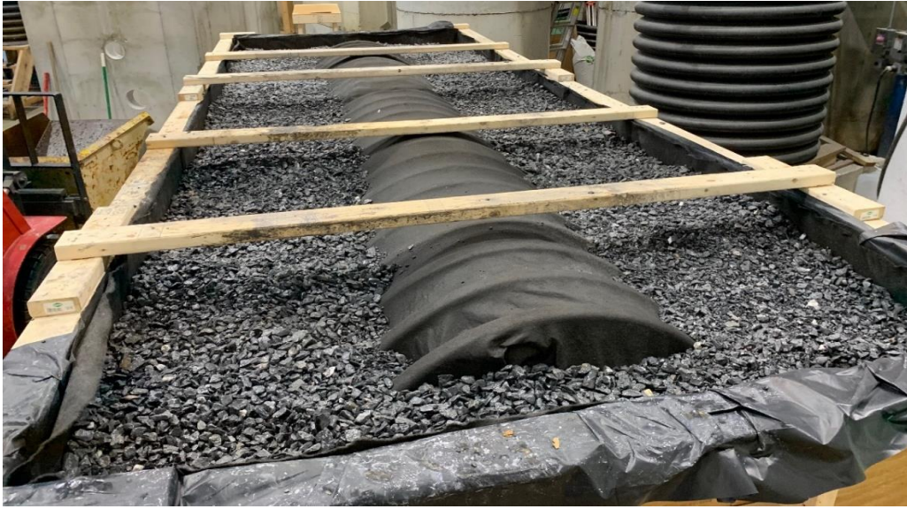
Figure 7 Top View Photograph of Isolator Row PLUS Test Box
