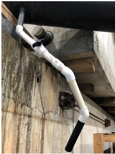
Figure 8 Photograph of Background Sampling Port
