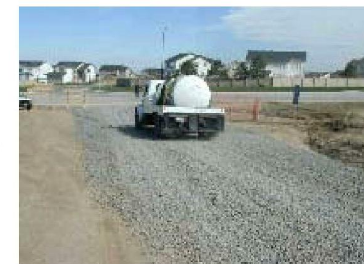
Photograph DC-1. Water truck used for dust suppression. Photo courtesy of Douglas County.
