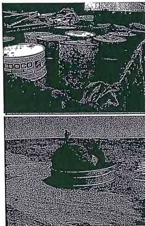
Photographs GH-1 and GH-2. Proper materials storage and secondary containment for fuel tanks are important good housekeeping practices. Photos courtesy of CDOT and City of Aurora.
