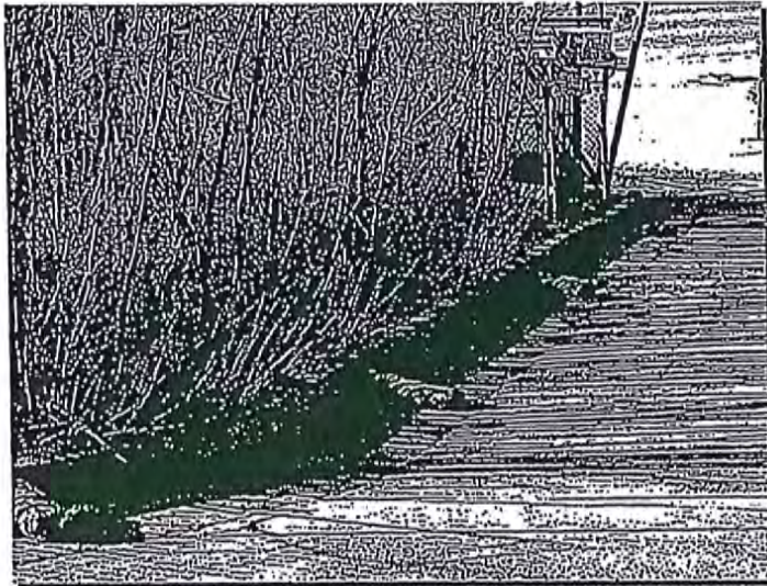
Photograph RS-1. Rock socks placed at regular intervals in a curb line can help reduce sediment loading to storm sewer inlets. Rock socks can also be used as perimeter controls.
