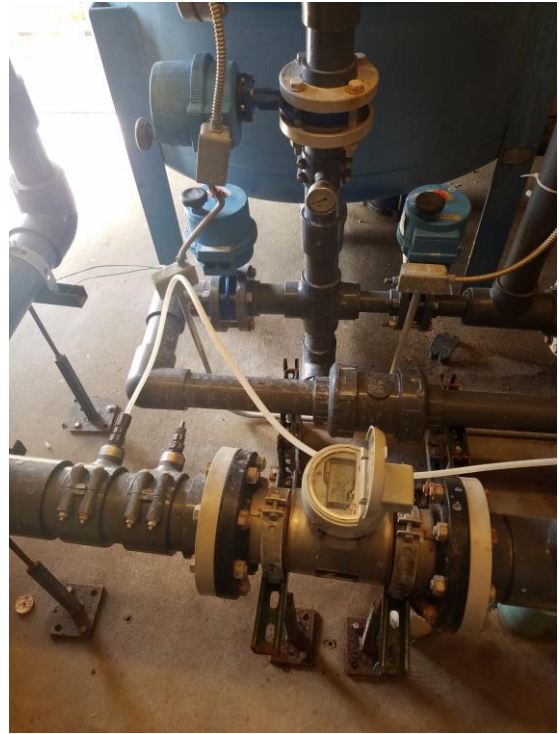
LFH2 Chlorine Addition
