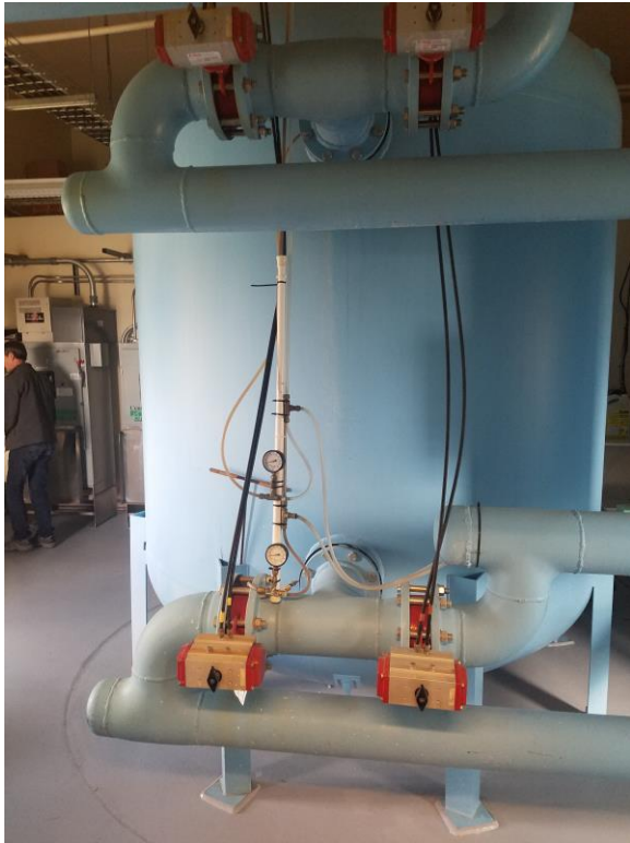
Filter and Control Valves
