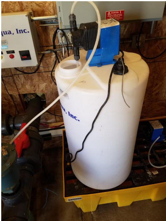
LFH2 Chlorine Storage and Pump
