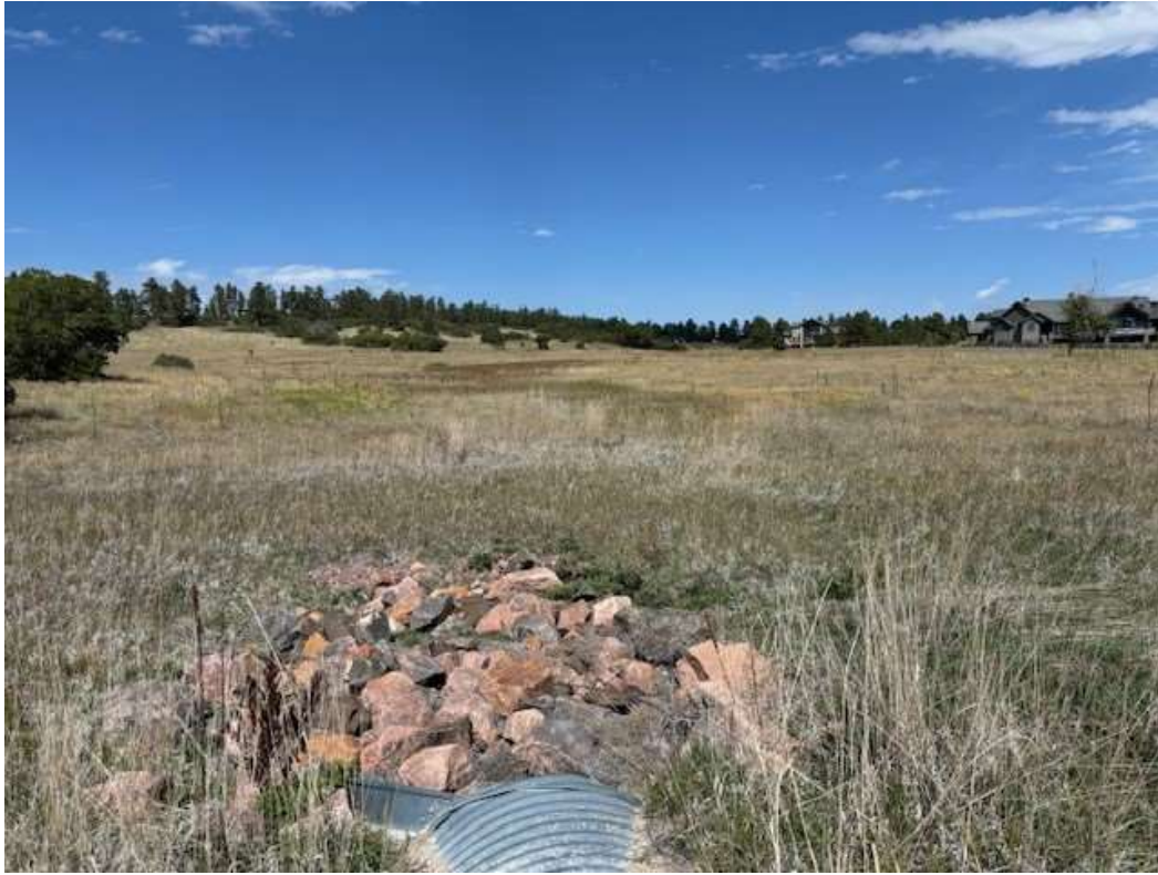
Existing Culvert P - 48" CMP Inlet with RR apron (facing NE; typical vegetation within Filing Three)
