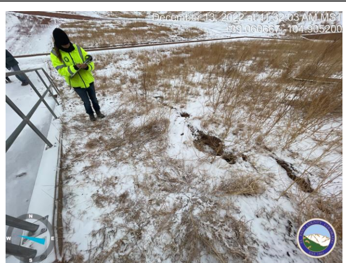
Photo 2: Erosion occurring on pond embankments
