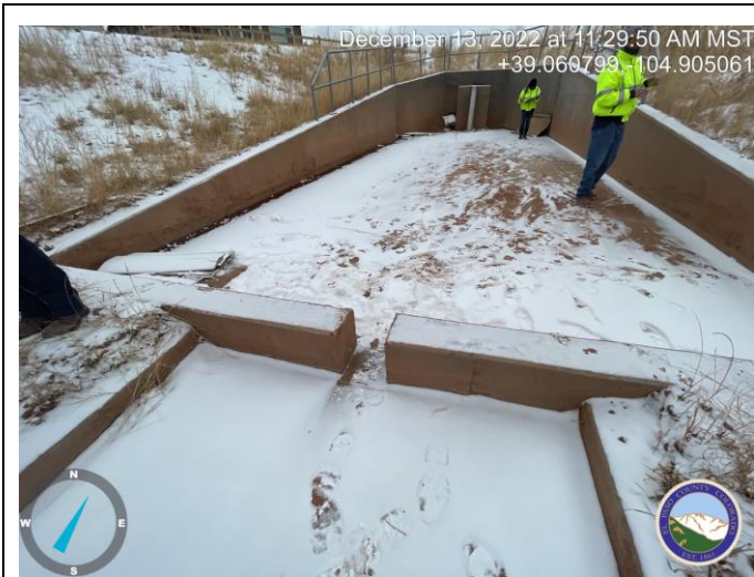
Photo 3: Forebay weir missing. Remove sediment from forebay.
