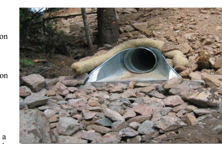
Photograph TOP-1. Riprap outlet protection.
