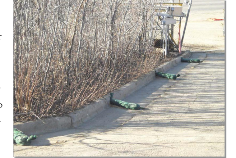
Photograph RS-1. Rock socks placed at regular intervals in a curb line can help reduce sediment loading to storm sewer inlets. Rock socks can also be used as perimeter controls.
