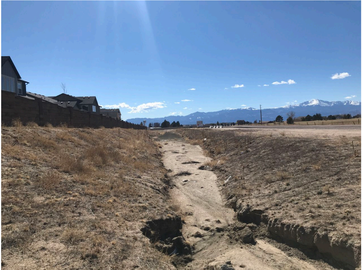
Photo Location 02. Looking south at drainage channel termination point. No apparent downstream connection to other aquatic resources.
