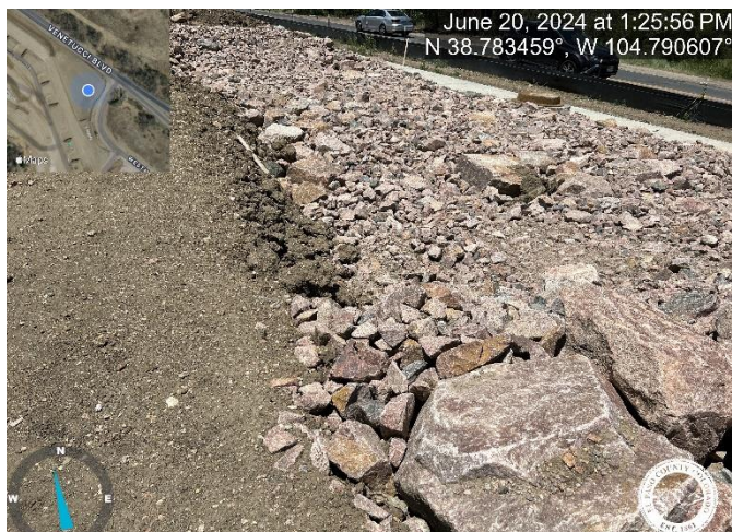
Photo 11: Either add top soil to rip rap per approved plans, or cut down soil to slope stated on plans.
