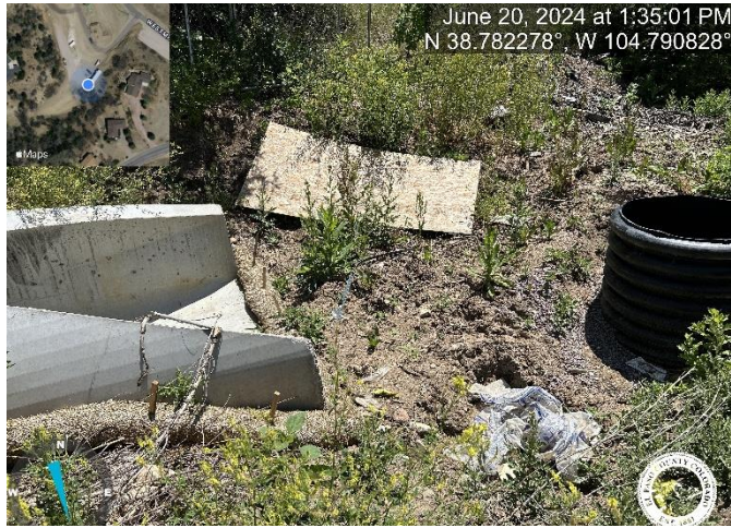
Photo 7: Fill in low spot near south outlet structure to allow positive drainage.
