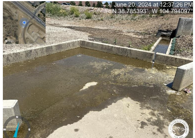
Photo 2: Raise pond bottom to top of trickle channel curb with a 3% slope towards trickle channel for positive drainage.
