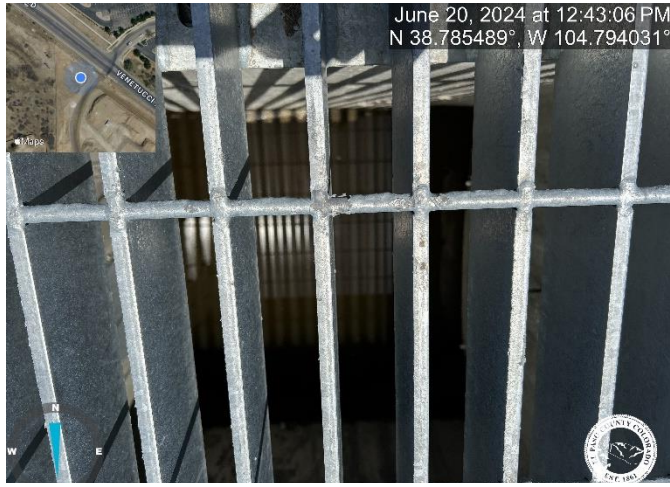
Photo 5: Steps are missing from inside the outlet structure. Install per approved plans
