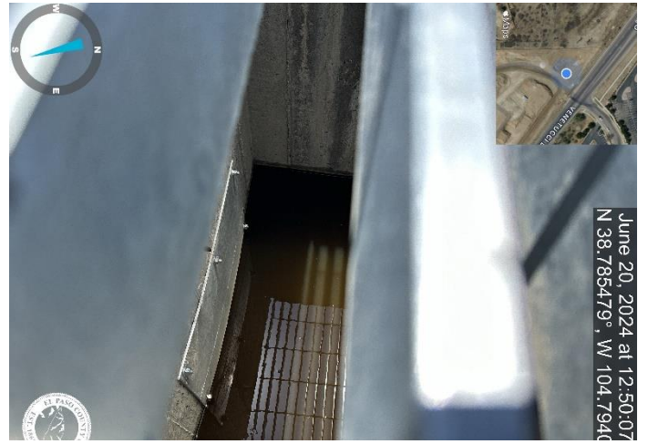
Photo 6: Standing water is pond bottom. Outlet Pipe is not visible due to it being covered in water. Possible clog somewhere between outlet structure and first manhole box along Venetucci.
