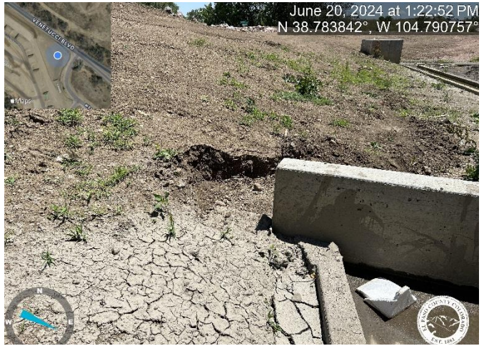
Photo 10: Water is bypassing.
