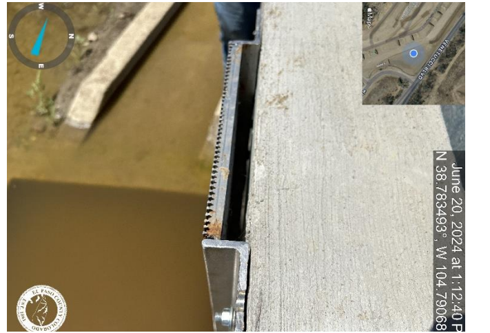
Photo 8: Eliminate gap above trash rack.
