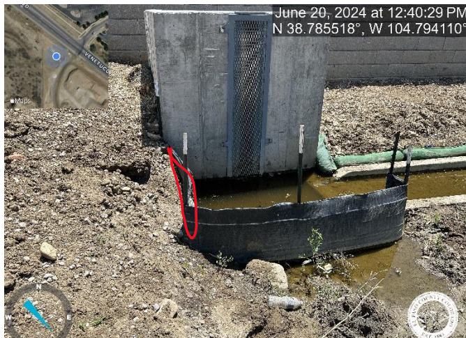
Photo 3: Regrade slope adjacent to micro pool to slope per plans. Remove silt fence.
