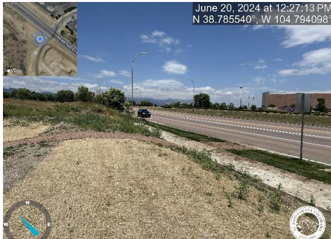
Photo 1: Concrete Driveway Apron is gravel instead of concrete as described on plans. Install per approved plans or confirm with your project engineer that this change from the plans is acceptable and then reflect the change on the as-builts.
