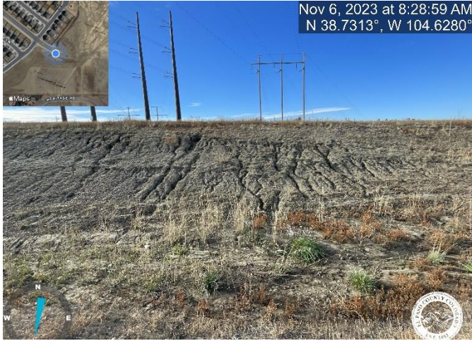
Photo 13: Swale 67a (east end of Trappe): Repair minor rilling and stabilize slope adjacent to area drain.
