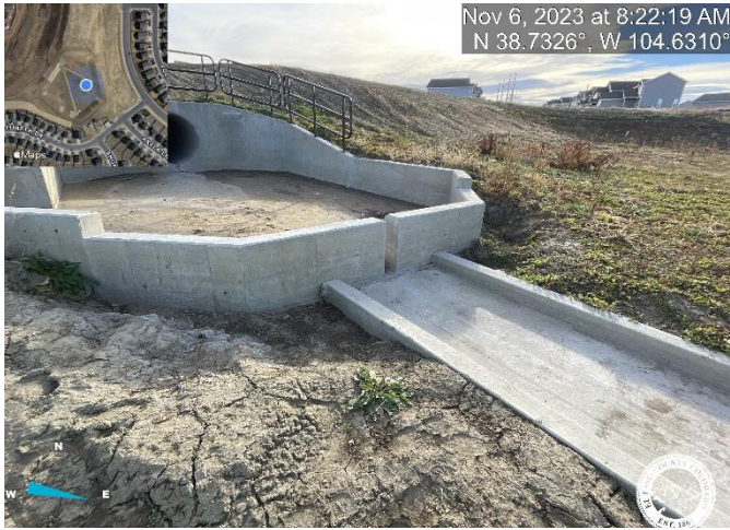
Photo 9: Confirm installation of 24" thick soil riprap at east forebay. Reference sheet C9.1 of the Construction Plans.
