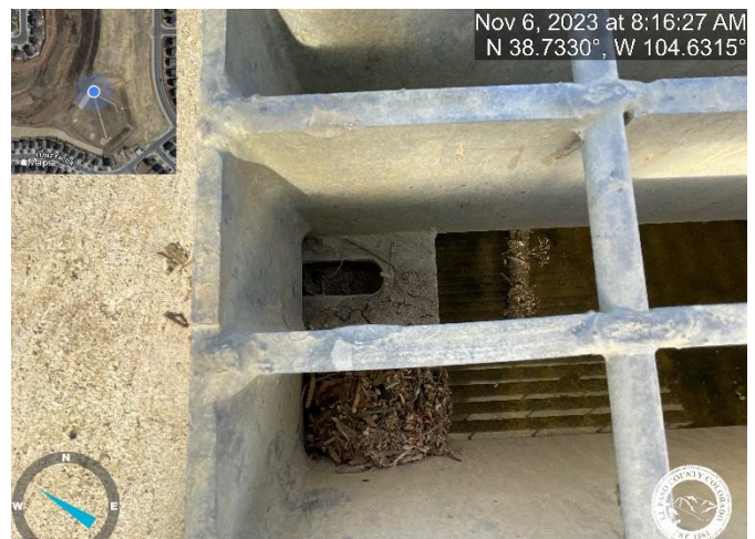
Photo 8: Implement missing bolts on outlet structure top grates.
