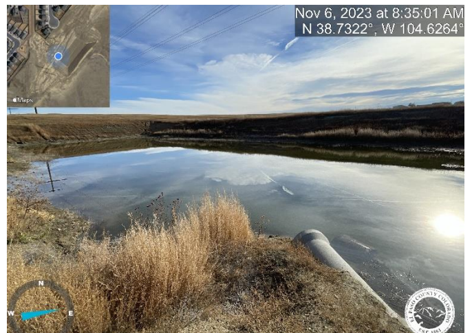
Photo 4: Implement missing low flow channel. Reference sheet C5.2 of the Final Grading and Erosion Control Plans.
