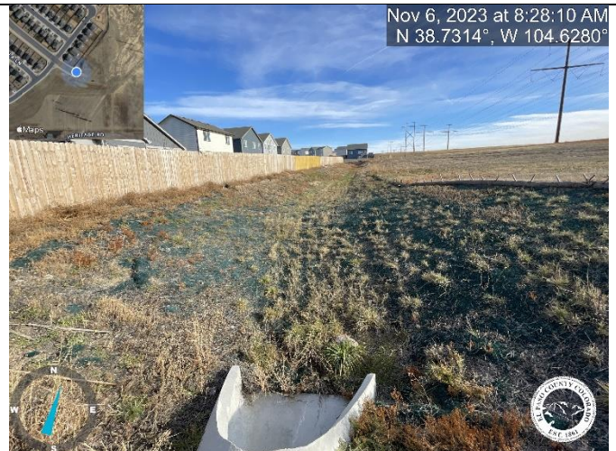
Photo 12: Swale 67b (east end of Trappe): Implement missing check dam (SD-3-62) or justify change within As-builts. Reference sheet C4.4 of the Final Grading and Erosion Control Plans.
