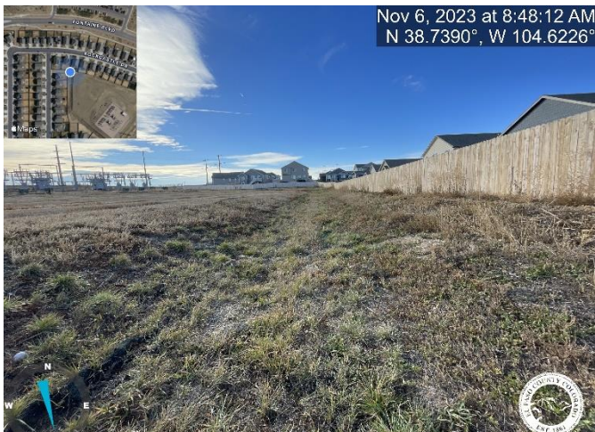
Photo 15: Substation Swale 2: Implement missing check dams (SD-3-62) or justify change within As-builts. Reference sheet C4.1 of the Final Grading and Erosion Control Plans
