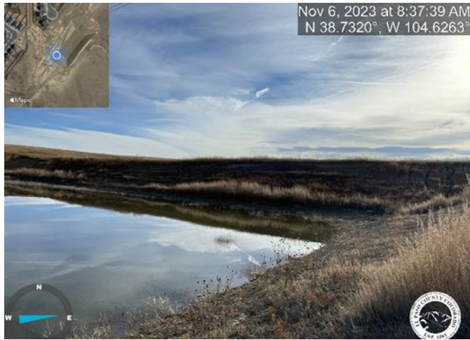
Photo 1: Implement missing AEC perimeter coconut fibernet or equivalent along the east perimeter slope. Reference sheet C5.2 of the Final Grading and Erosion Control Plans.
