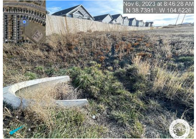
Photo 14: Substation Swale 2: Implement missing 9" D50 riprap 18" thick on fabric at RCP inlet or justify change in As-builts. Reference sheet C7.1 of the Construction Plans.
