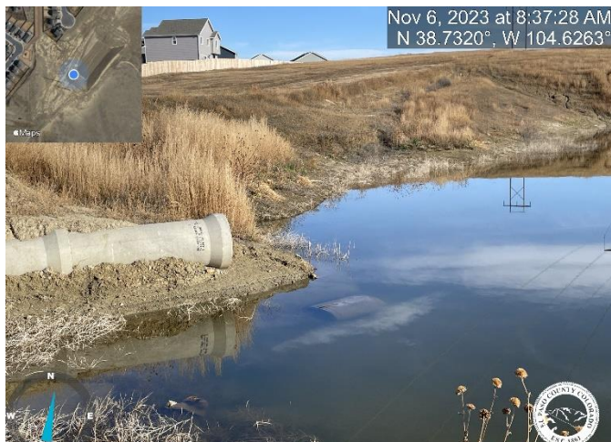
Photo 3: Implement missing 12" high riprap check dam with fabric and riprap pad at outlet pipe. Reference sheet C5.2 of the Final Grading and Erosion Control Plans.
