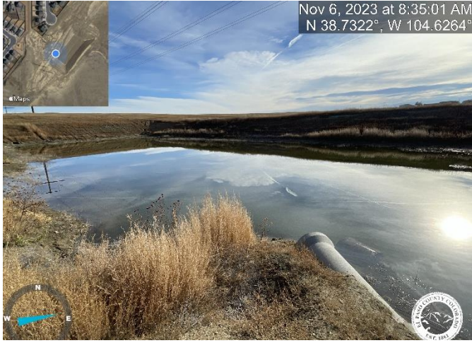
Photo 5: Water retention within pond. Fill pond bottom to be at approved grade to allow for positive drainage.
