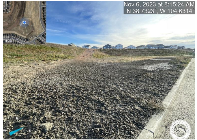
Photo 10: Remove excess sediment from maintenance access road within pond bottom and reestablish road base along trickle channel. Access road should consist of 12" thick class 6 aggregate. Reference sheet C9.1 of the Construction Plans.
