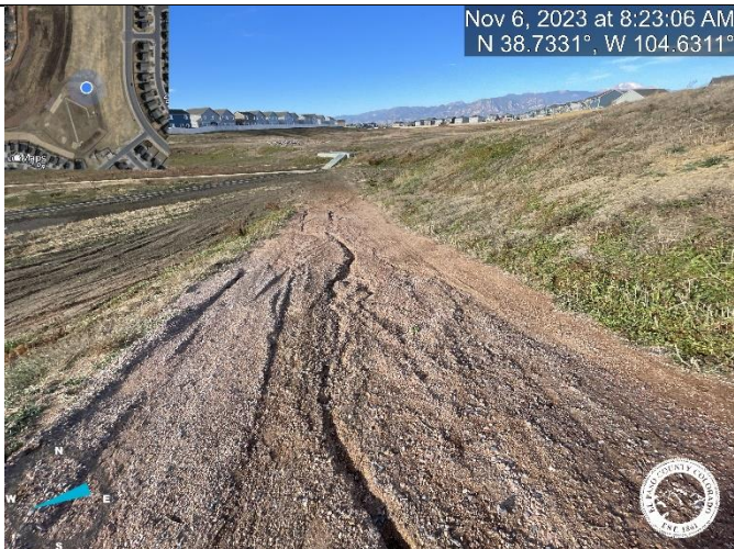
Photo 11: Repair rilling along maintenance access road. Rilling could worsen and will be required to be repaired at Final Acceptance.
