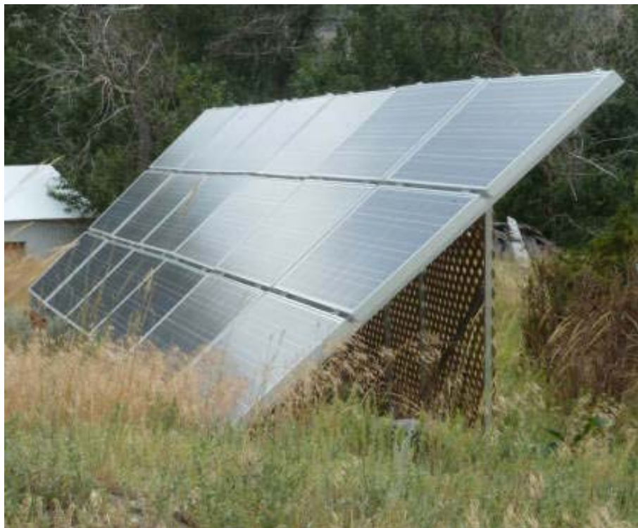
Photo 4. Non-acceptable vegetation management
