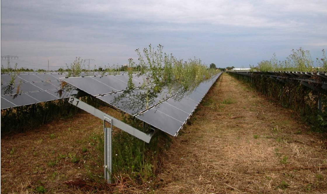
Photo 3. Non-acceptable vegetation management
