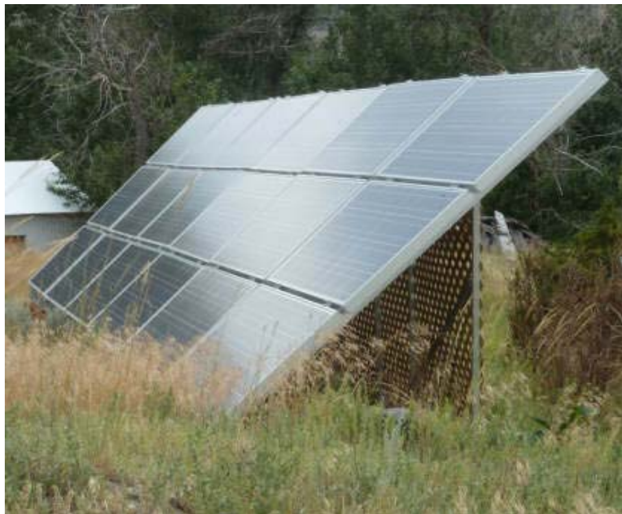
Photo 4. Non-acceptable vegetation management
