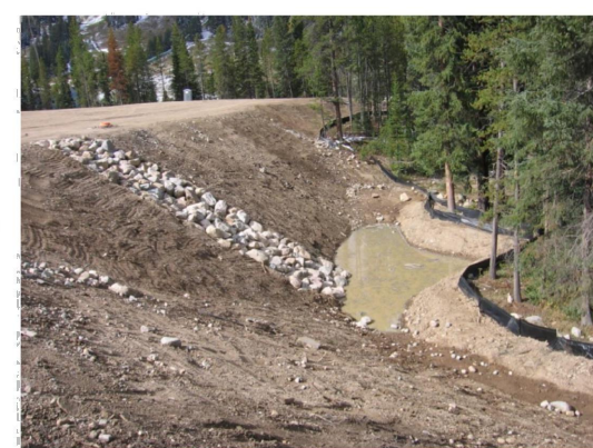
Photograph SB-1. Sediment basin at the top of a slope. Photo courtesy of UDFCD.
