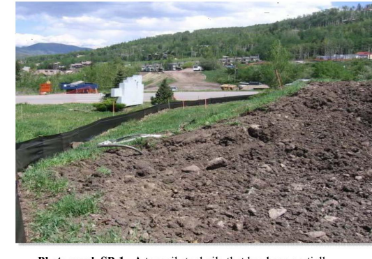
Photograph SP-1. A topsoil stockpile that has been partially revegetated and is protected by silt fence perimeter control.
