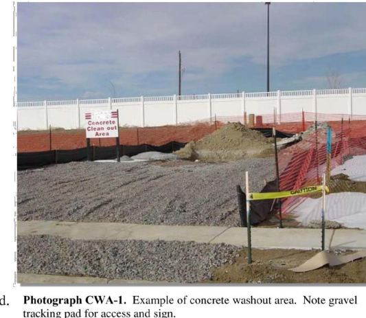
Photograph CWA-1. Example of concrete washout area. Note gravel tracking pad for access and signs.
