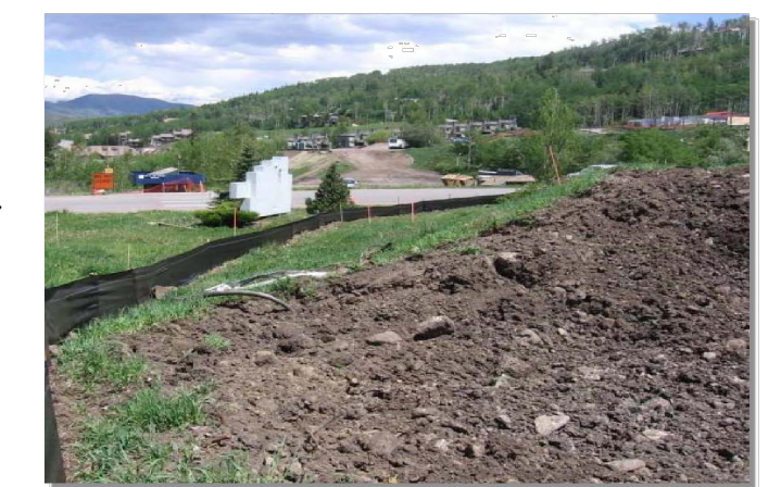
Photograph SP-1. A topsoil stockpile that has been partially revegetated and is protected by silt fence perimeter control.
