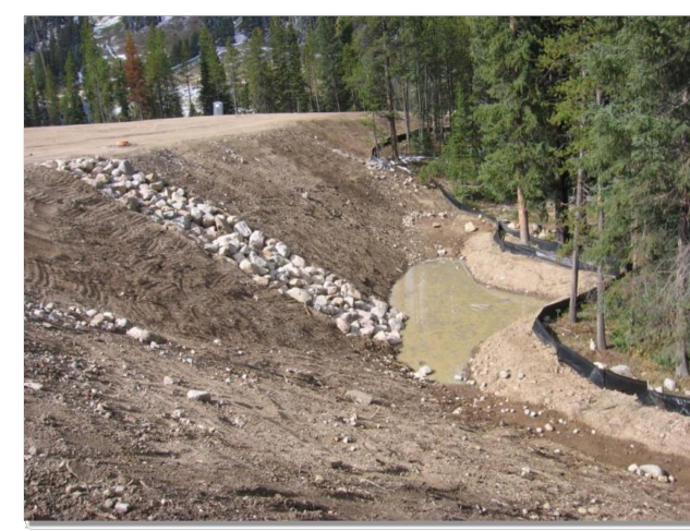
Photograph SB-1. Sediment basin at the toe of a slope. Photo courtesy of WVE.
