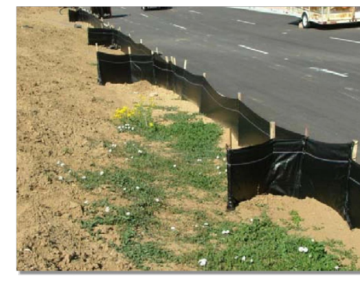
Photograph SF-2. When silt fence is not installed along the contour, a "J-hook" installation may be appropriate to ensure that the BMP does not create concentrated flow parallel to the silt fence. Photo courtesy of Tom Gere.
