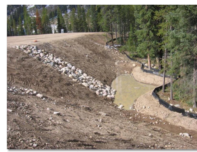
Photograph SB-1. Sediment basin at the toe of a slope. Photo courtesy of WWF.
