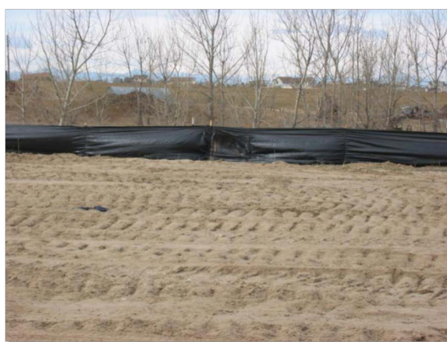
Photograph SF-1. Silt fence creates a sediment barrier, forcing sheet flow runoff to evaporate or infiltrate.
