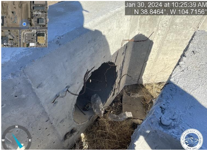
Photo 5: Pond B: Remove exposed wire from forebay B2.
