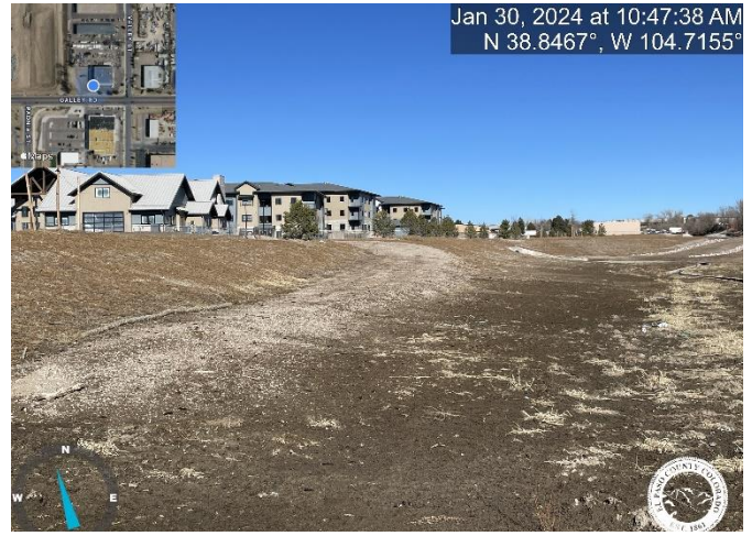
Photo 6: Pond B: Maintenance access should be flush with the grade at a 2% slope. Maintenance access road should be 15' in width. Reference Sheet 22 of the Construction Drawings.
