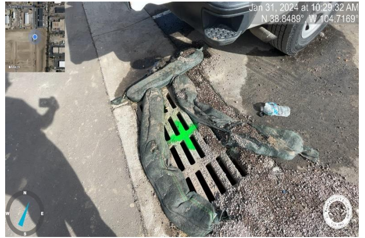
Photo 26: Area drain inlets that need to be cleaned of sediment and debris are marked with green paint on the grate (photo is an example of marked inlet).
