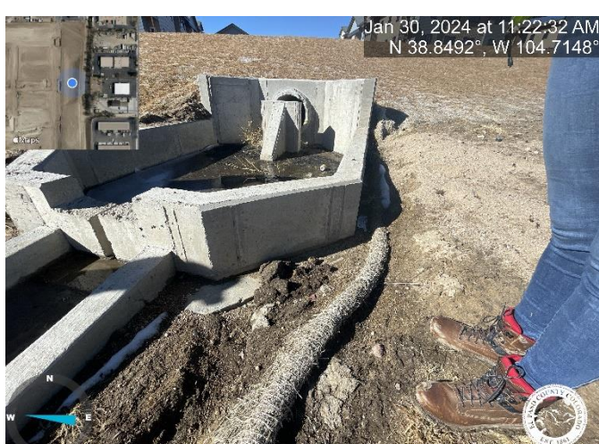
Photo 19: Pond A: Fine grade rill erosion around forebay and stabilize.
