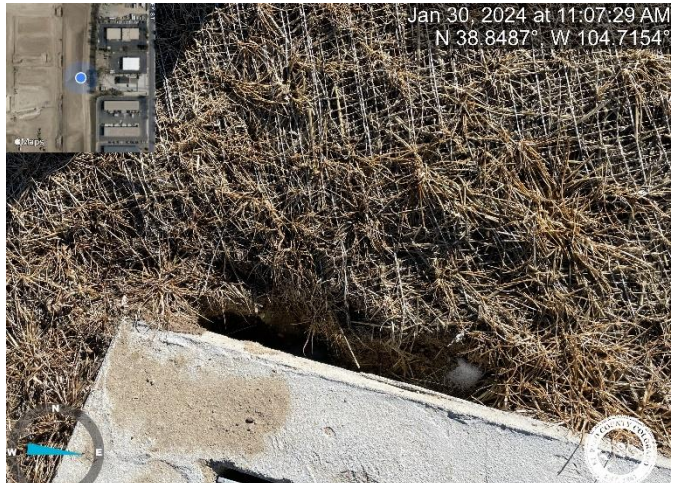
Photo 14: Pond A: Fine grade rill erosion behind the outlet structure and stabilize.
