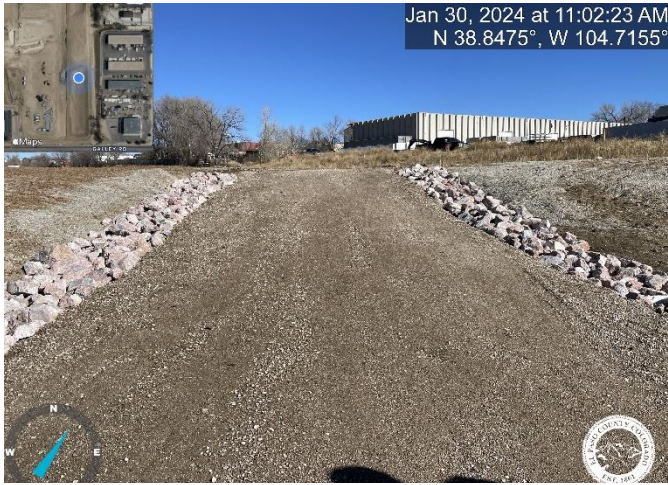
Photo 9: Pond B: Confirm installation of 8" class 6 aggregate base course or 12" class 6 aggregate base course. Reference Sheet 22 of the Construction Drawings.
