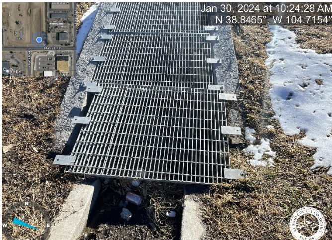
Photo 11: Pond B: Failure to install properly sized trash racks. Reference Sheet 23 of the Construction Drawings.
