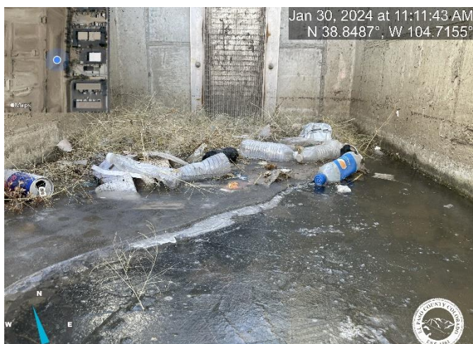
Photo 15: Pond A: Micropool is not holding water to the invert of the bottom hole on the orifice plate. This indicated that the orifice plate does not have a watertight seal.
