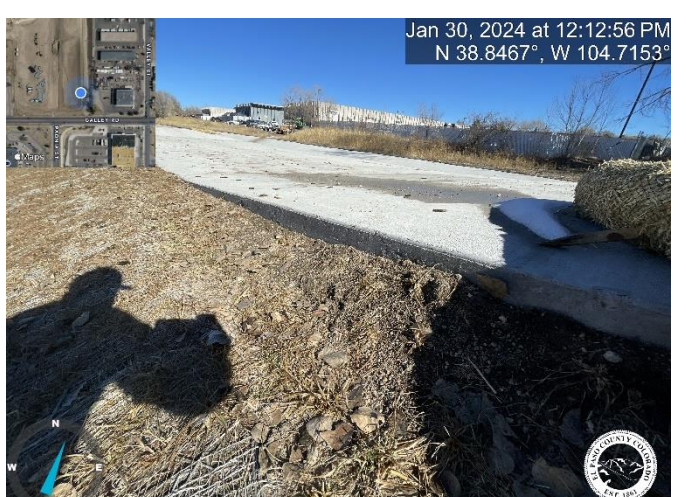
Photo 20: Pond B: Raise grade to be flush with the Emergency Overflow Spillway.
