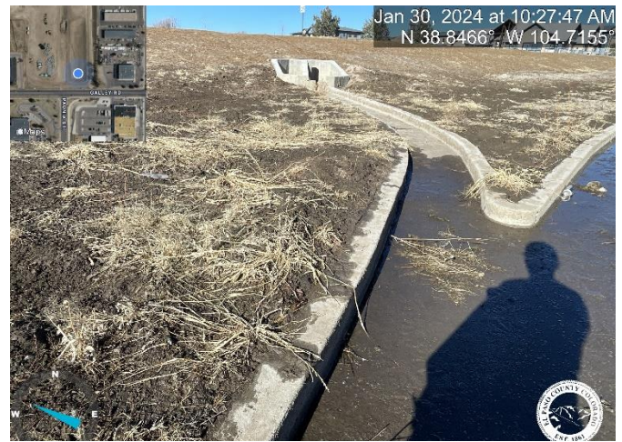
Photo 2: Pond B: Grade Pond bottom to be flush with the top of the trickle channel curb with a 3% slope towards trickle channel for positive drainage.
