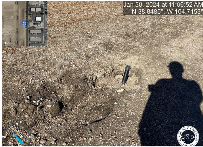
Photo 13: Pond A: Fine grade rill erosion behind the outlet structure and stabilize.
