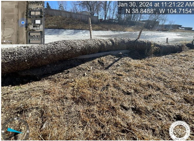
Photo 21: Pond A: Raise grade to be flush with the Emergency Overflow Spillway.
