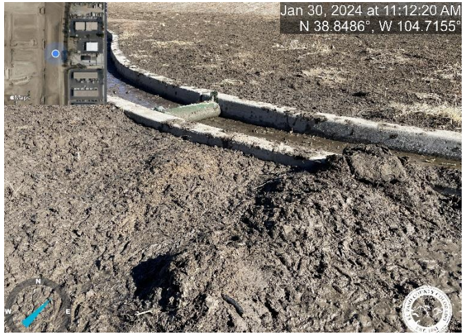
Photo 18: Pond A: Grade Pond bottom to be flush with the top of the trickle channel curb with a 3% slope towards trickle channel for positive drainage.
