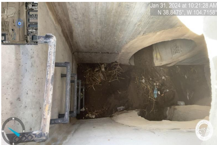
Photo 23: Example of inlet that needs to be cleaned.
