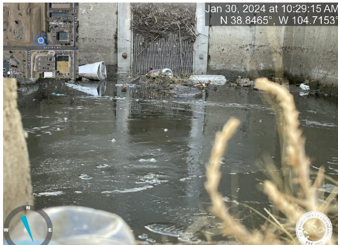
Photo 12: Pond B: Micropool is not holding water to the invert of the bottom hole on the orifice plate. This indicated that the orifice plate does not have a watertight seal.
