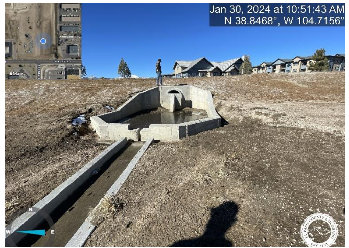
Photo 8: Pond B: Fine grade rill erosion around forebay B1 and stabilize.
