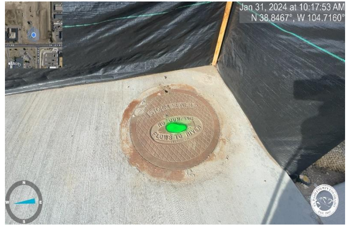
Photo 22: Inlets that need to be cleaned of sediment and debris are marked with green paint on manhole lid (photo is an example of marked inlet).
