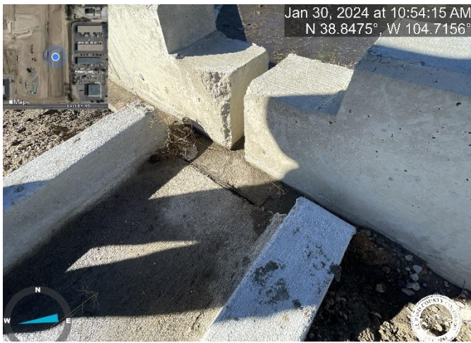
Photo 7: Pond B: Extend trickle channel to be flush with forebay B1.
