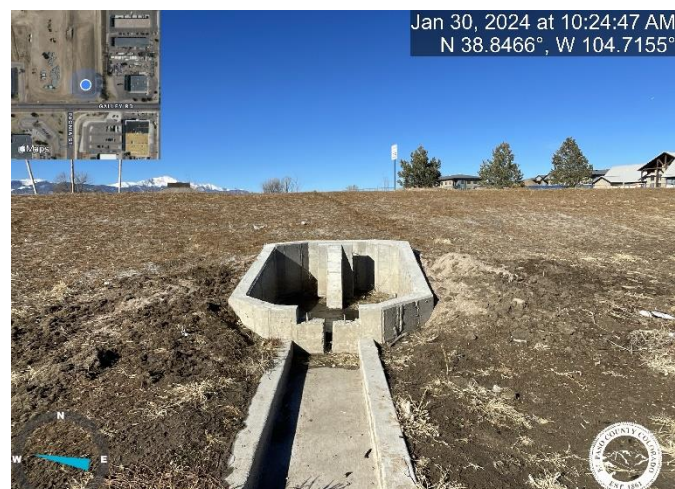
Photo 3: Pond B: Fine grade rill erosion around forebay B2 and stabilize.
