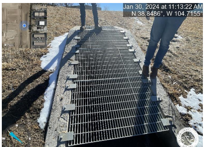
Photo 16: Pond A: Failure to install properly sized trash racks. Reference Sheet 19 of the Construction Drawings.
