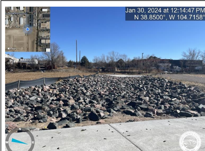
Photo 1: Overflow channel: Plans call for 24" deep Type M Soil Riprap. Reference sheet 4 of the channel Improvement plans.
