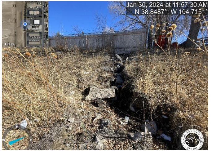
Photo 6: Approximately STA 11+00: Fine grade rill erosion along slope and stabilize.
