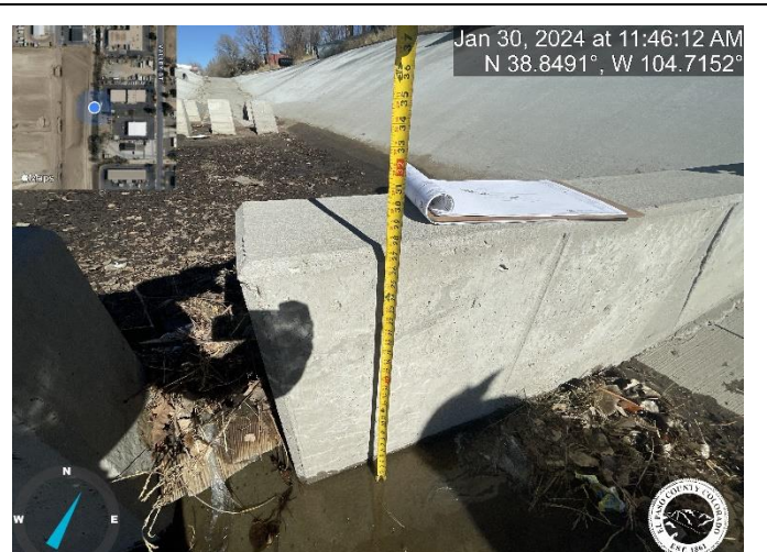
Photo 4: Concrete Sill Wall at STA 13+05 deviates from approved design. Plans call for a height of 2.25'. Reference deviation on the As-builts.
