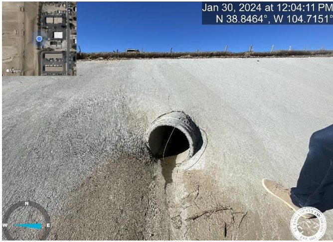
Photo 7: Ponds A and B: Plans call for a flared end section at outlet pipe from the ponds. Reference deviation on the As-builts.
