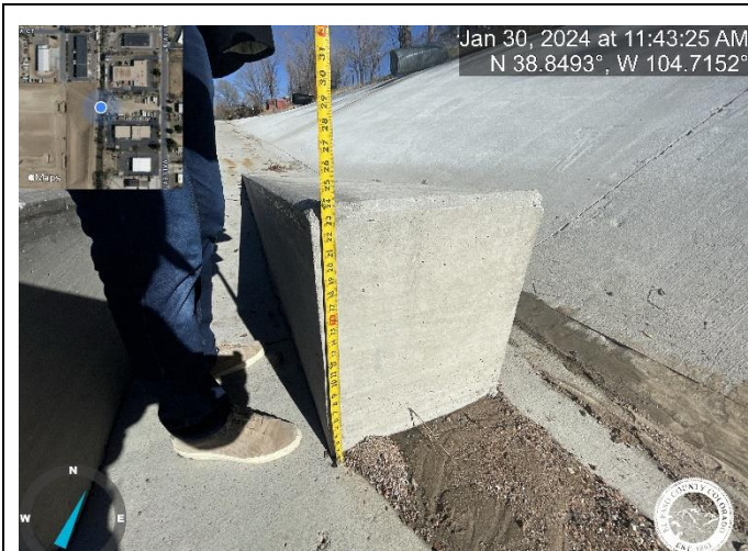
Photo 3: Concrete Baffle Blocks deviate from approved design. Plans call for a height of 1.68'. Reference deviation on the As-builts.
