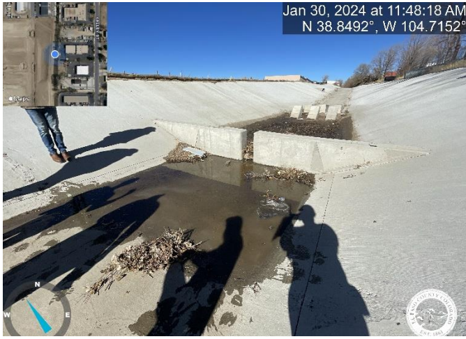
Photo 5: Approximately STA 13+00: Low spot is causing water accumulation. Adjust grade to match the approved 1% slope to promote positive drainage.
