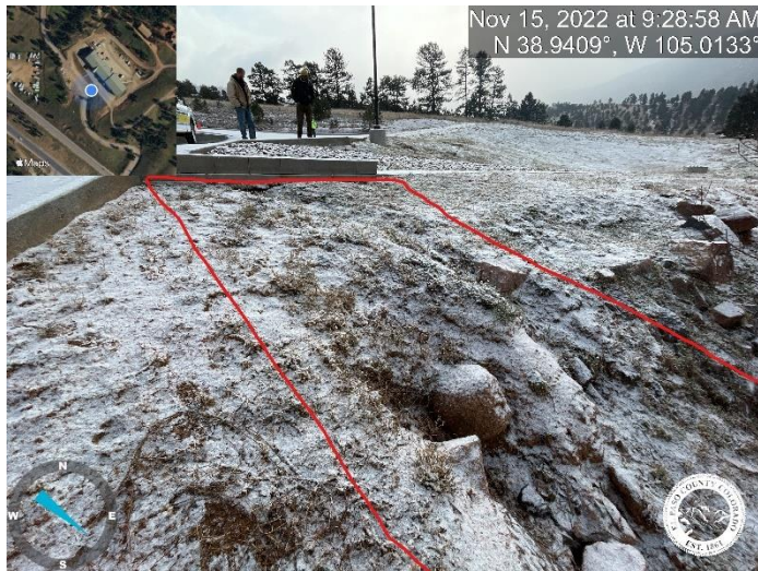
Photo 11: East detention pond; Address erosion behind cinderblocks above STA 1+26.61.
