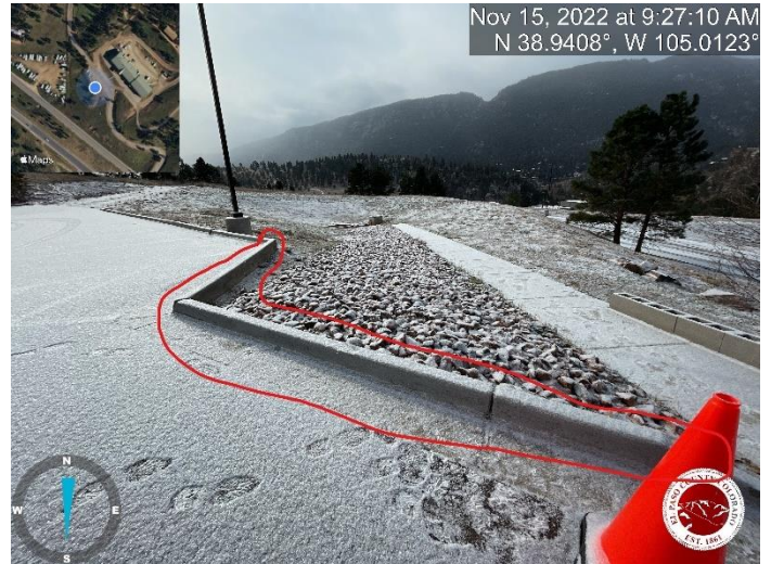
Photo 10: East detention pond; Remove curb to allow access to the gravel maintenance road as depicted on C2.9 of the Erosion Control Plans.
