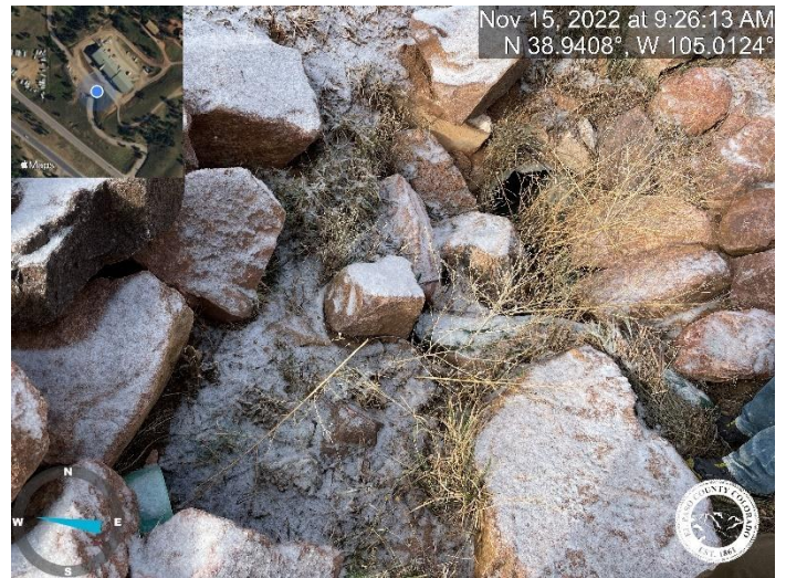
Photo 12: East detention pond outlet at STA 1+26.61. Remove sediment and debris to allow for positive drainage.
