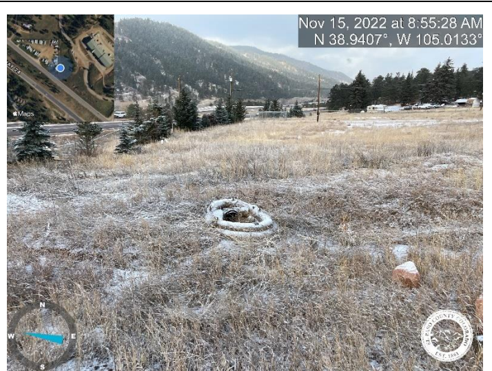
Photo 2: Remove all temporary control measures throughout site. Photo depicts straw wattle near STA 2+22.54.
