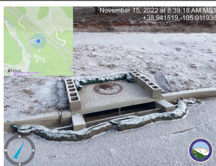
Photo 1: Remove inlet protection, as well as the 2x4 forms inside the inlet at STA 0+07.50.
