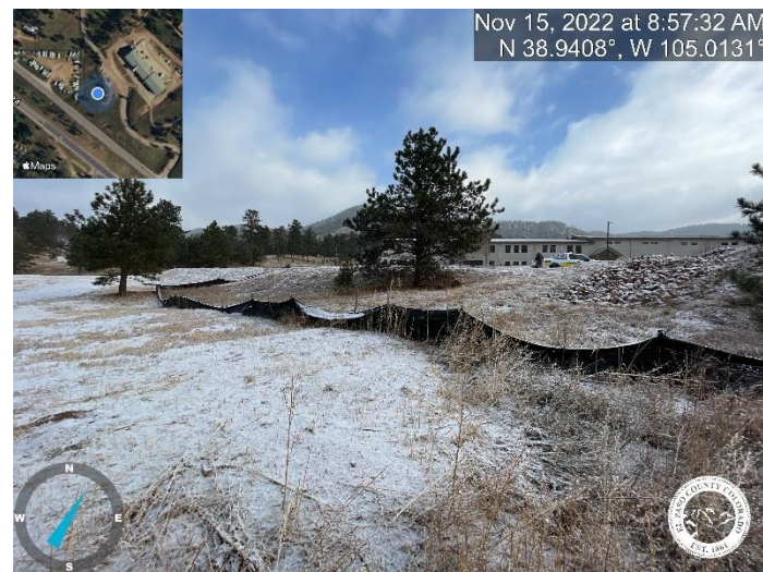
Photo 3: Remove all temporary control measures throughout site. Photo depicts silt fence below the west detention pond.
