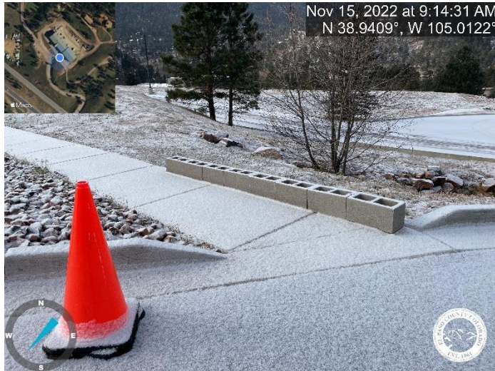
Photo 9: East detention pond; Remove temporary cinderblocks and replace with a permanent control measure (e.g., cement curb)
