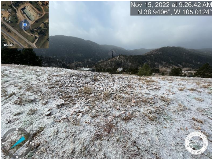
Photo 13: East detention pond; Emergency overflow path is not installed per detail. Provided detail on Sheet C2.9 shows that the path should measure 18' at the base.
