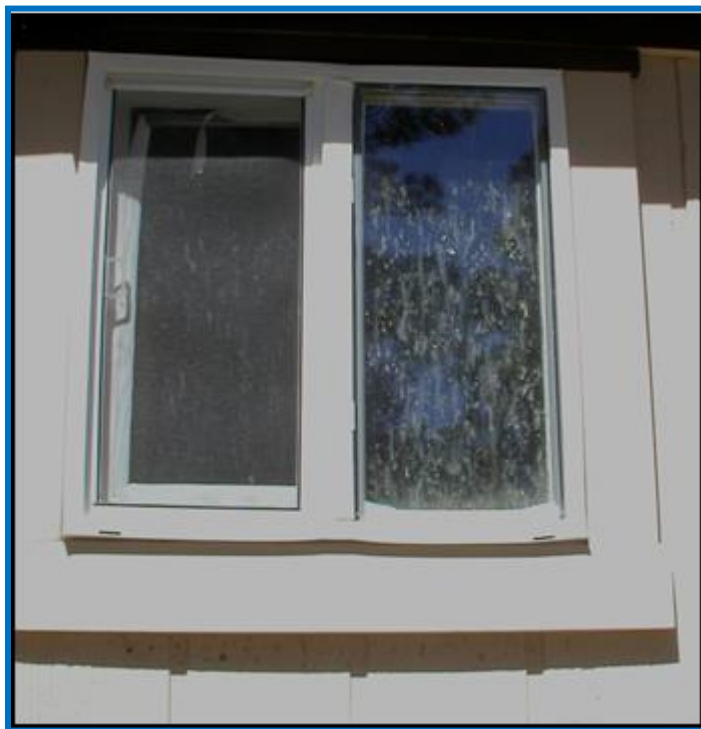
The vinyl window frame on this home melted and warped in the Black Forest Fire, but not enough to allow firebrands inside the home. Metal framed windows resist warping.
