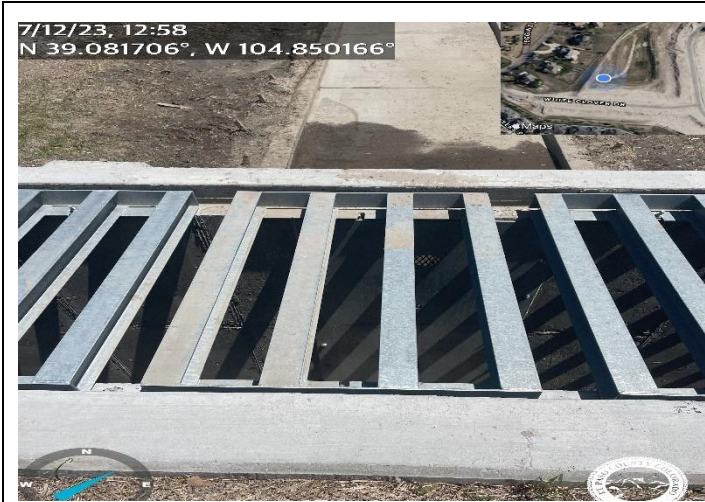
Photo 1: Pond P2 missing bolt above 42" RCP above trash-rack.
