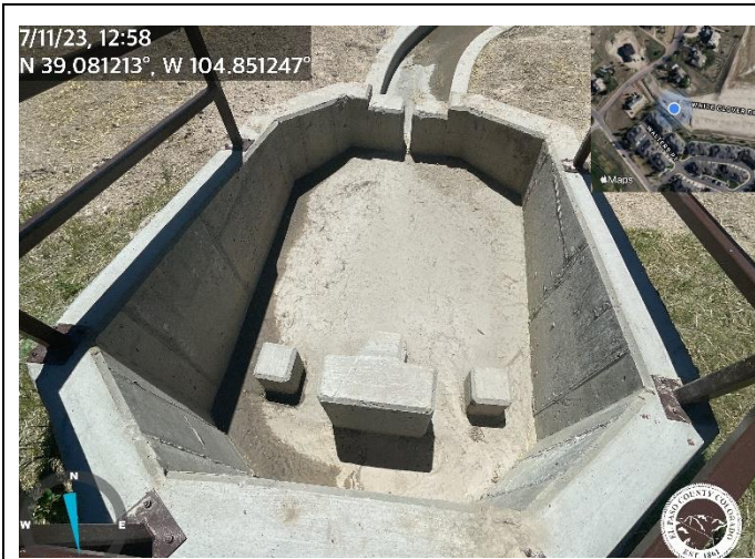
Photo 3: Pond 4 Forebay is missing 4 secondary baffle blocks. Submit as-builts to show that this is acceptable.
