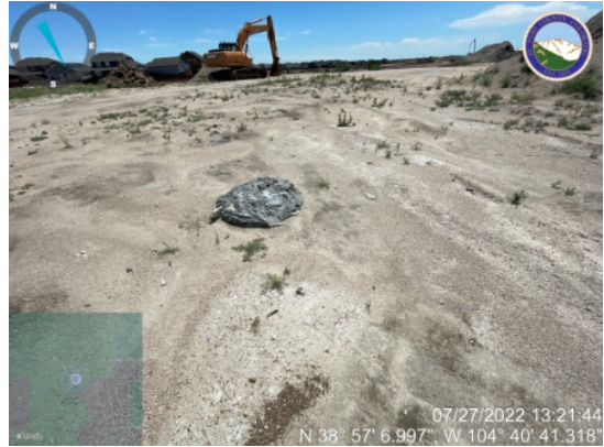
Properly dispose of cured concrete and implement CWO near pond 5.
