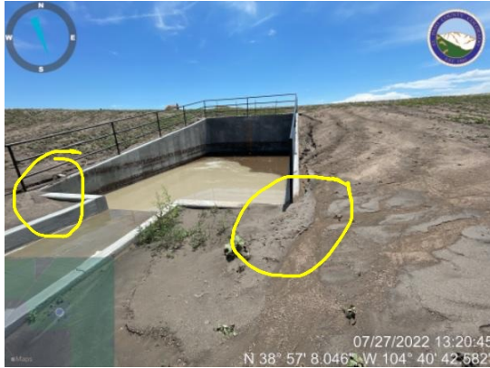
Implement control measures to prevent sediment from entering water quality pond 5 at outlet structure.
