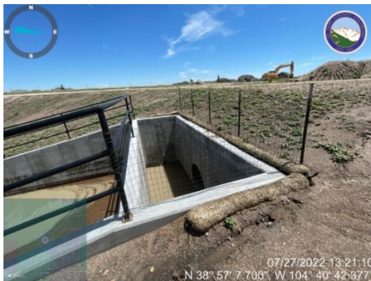
Ensure straw wattle control measure is staked down as per detail at WQ pond 5.
