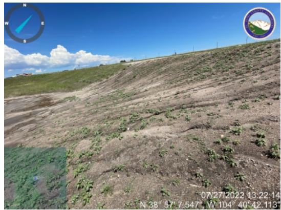
Extend ECB stabilization matting to encourage vegetative establishment along embankment at WQ pond 5.
