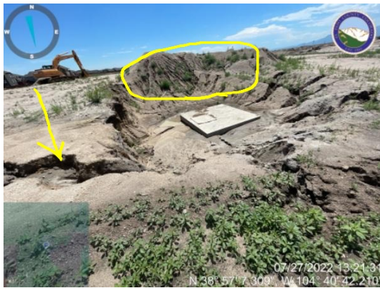
Address gully formation and unprotected stockpile at Box up gradient of WQ pond 5.
